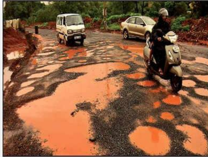
Poor roads condition
